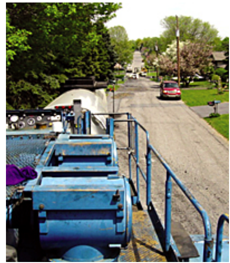
This view from the top of the recycling machine shows the condition of the roadway: worn pavement, top-down cracking, and multiple pothole patches.
