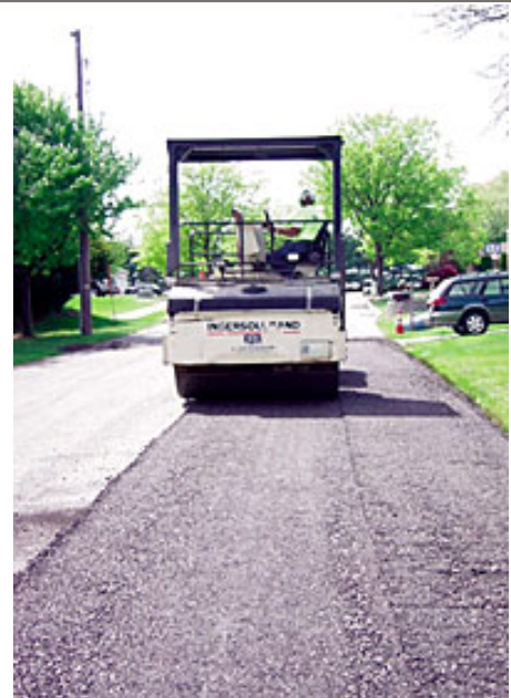
A tandem steel-wheel roller compacts the recycled pavement. After a two-week curing period, the township places a hot-mix overlay on the new base.
