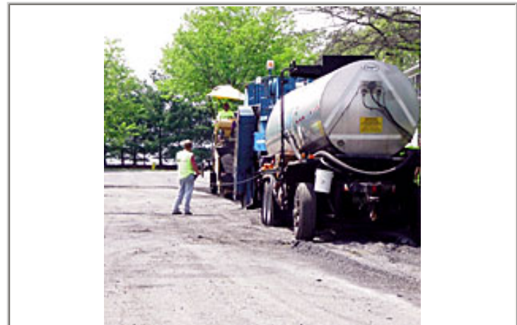
E.J. Breneman's compact cold-in-place recycling train processes the aged asphalt of a Bethlehem Township residential street into a rejuvenated base.
