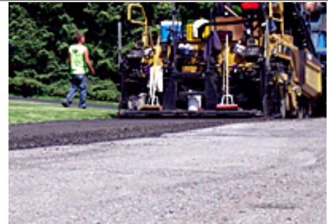
Breneman uses a hot-mix asphalt paver to place the cold-processed recycled pavement coming from the main recycling machine.
